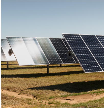
Our Maiden, North Carolina data center is powered by our biogas fuel cells and three solar arrays.
