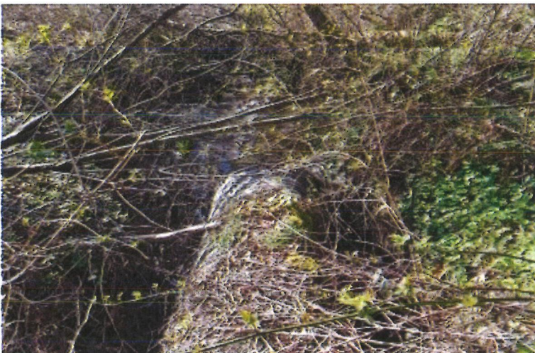
Photo 4 was taken from the same location as Photo 3. The culvert is plugged with debris, so the stream channel has widened around the culvert and eroded some of the soil around it.
