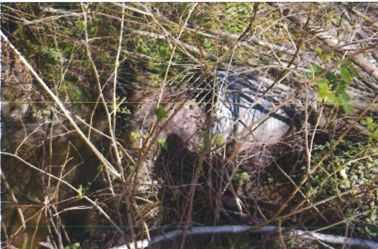
Photo 5 shows the opening of the culvert. A trash rack covers the opening and is clogged with debris. The culvert continues underground and day-lights approximately 445 feet to the north. Fish passage appears to be impossible through the clogged culvert.
