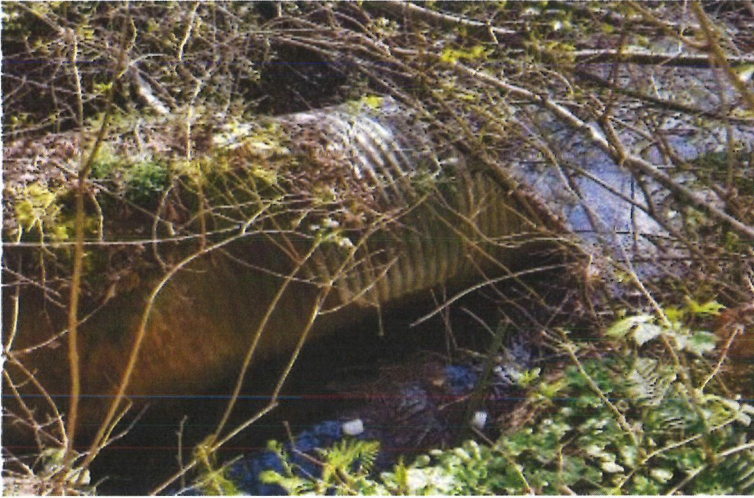
Photo 3 was taken approximately 67 feet south of the southern lot line where a large culvert, approximately 5 feet in diameter, is present. A stream, which flows to the north, enters this culvert.
