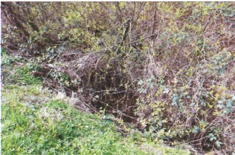
Photo 11 was taken near the outlet of the culvert looking west where the stream daylights, approximately 445 feet north of the culvert inlet. A culvert begins at the end of this stream and conveys water under Bethel Road.
