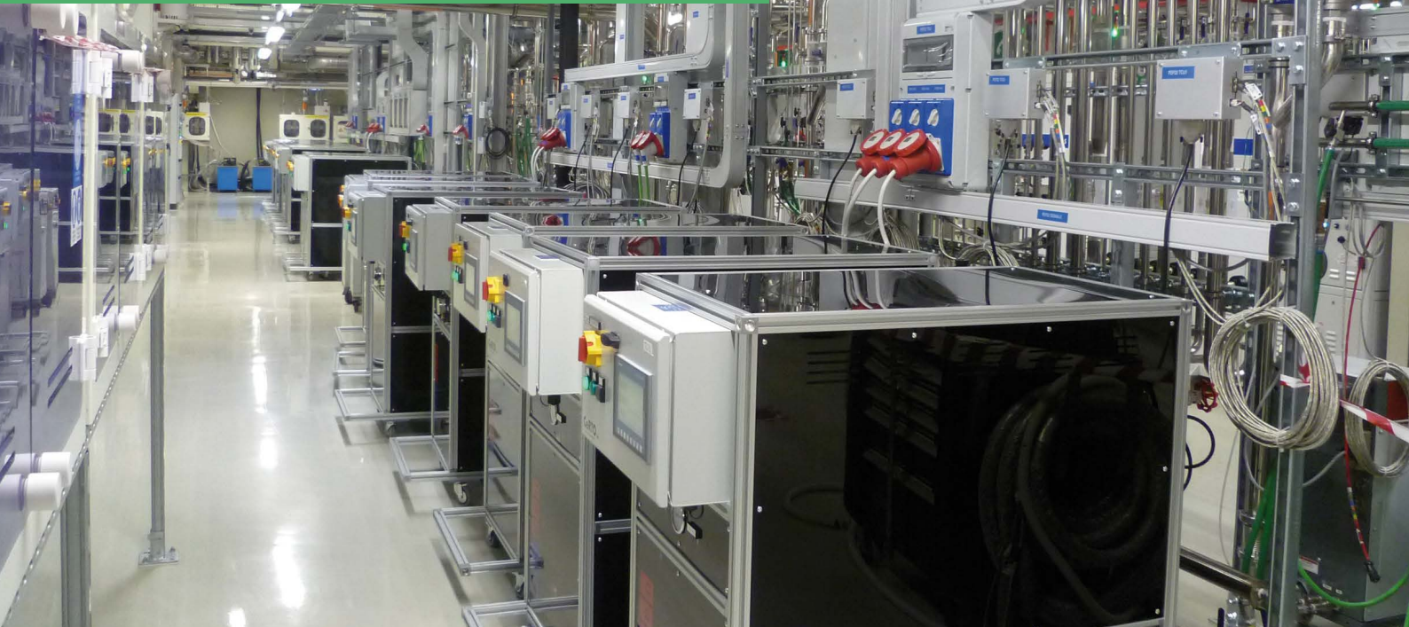
Thermal processing units, ST Catania, Italy
