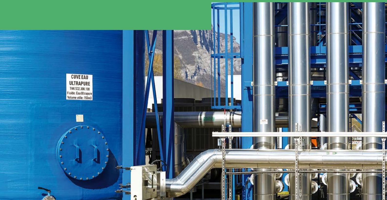
Ultra-pure water, ST Crolles, France
