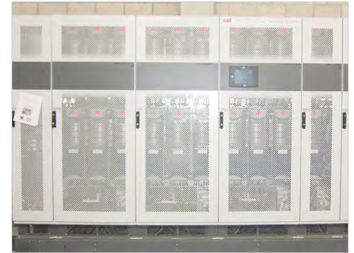
Providing grid interconnection from 50 Hz to 60 Hz
