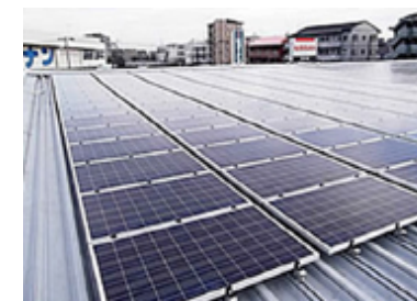
Solar panels installed on the roof of a Kanagawa Nissan dealership. Power from the panels is supplied to dealerships through the Nissan PPS system.
