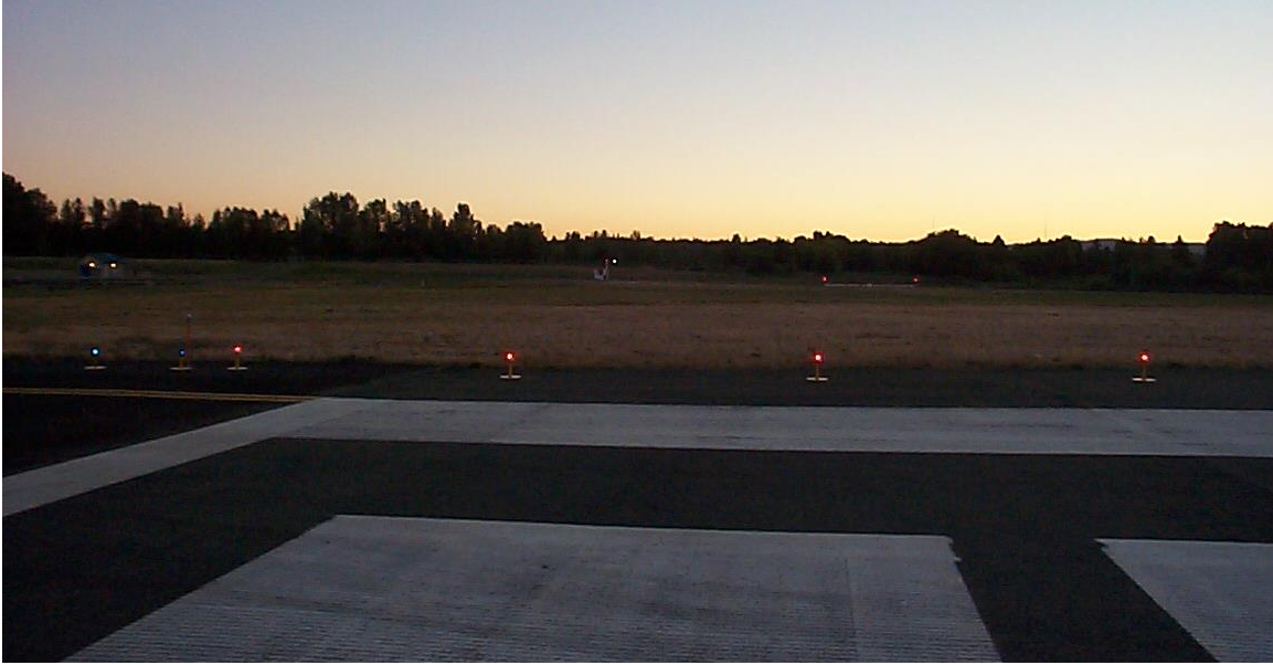
Runway End Lights
