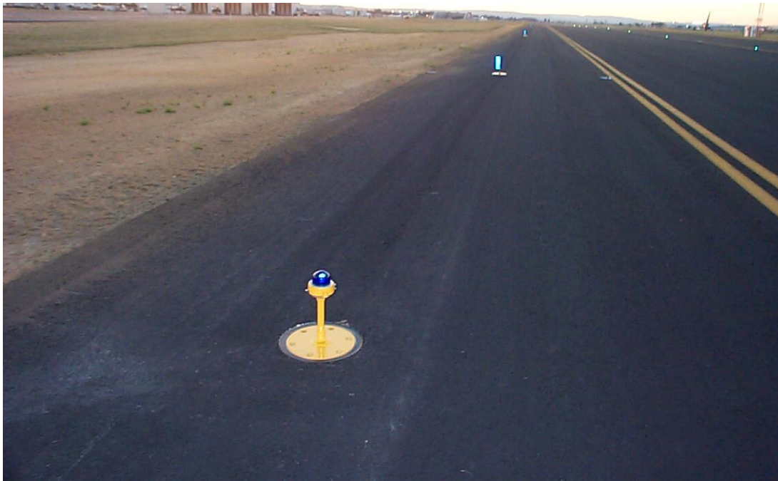
Taxiway edge light, Taxiway edge reflector and Green taxiway centerline lights
