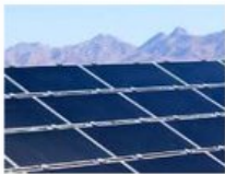
Yuma Foothills Solar 35 MW
