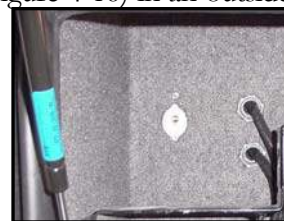
Figure 4-16. Cable & Telephone Jack
