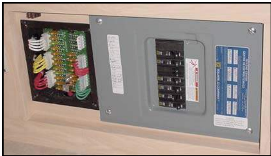
Figure 7-1. Circuit Breaker Box
