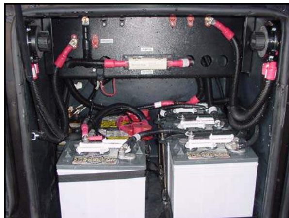
Figure 7-5. 12 VDC Battery System
