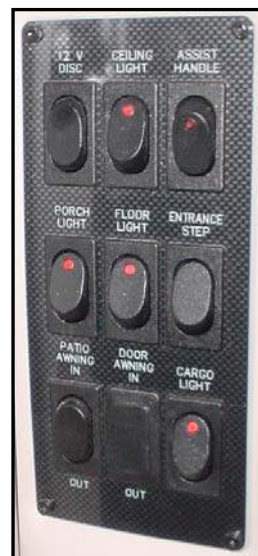
Figure 7-8. 12 VDC Disconnect Switch
