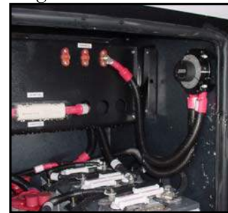
Figure 7-7. House Battery Disconnect Switch (right side)
