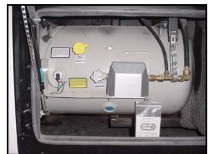
Figure 3-4. Liquid Propane Tank
