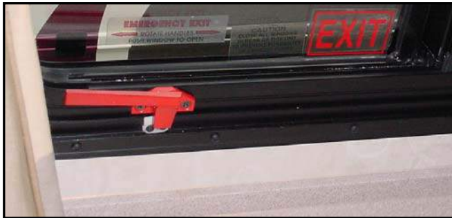
Figure 13-2. Bedroom Emergency Exit Window
