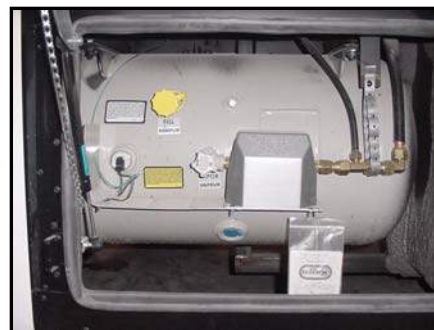
Figure 2-4. Liquid Propane Tank
