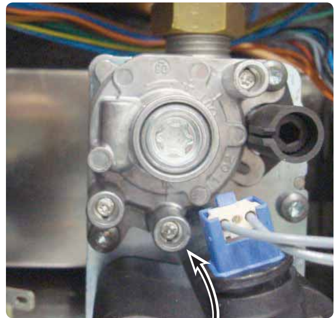
Figure 60 Inlet test port on gas valve
