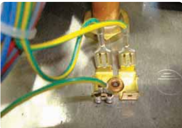
Figure 138 Ignition electrode grounding
