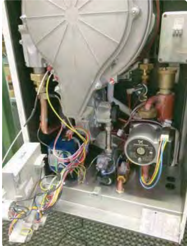
Figure 139 Boiler front panel removed
