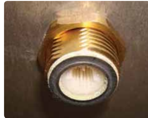
Figure 43 DHW inlet has a filter screen
