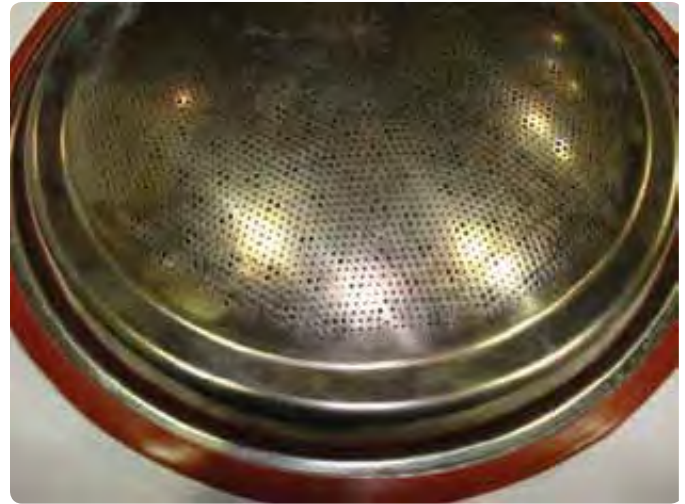
Figure 143 Inspecting exterior and cleaning the burner
