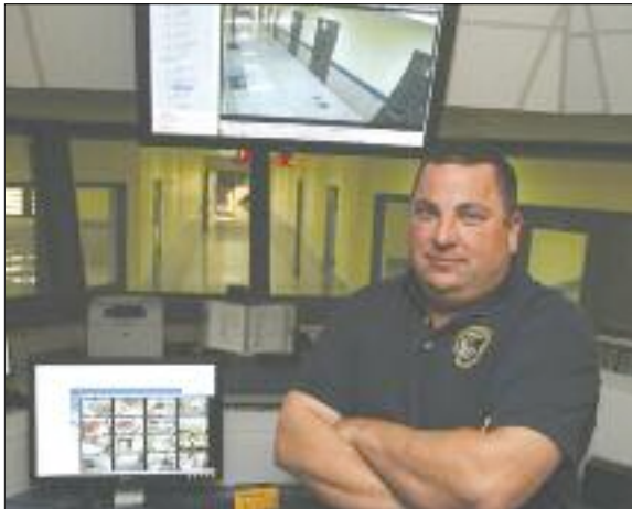
As security auditor for Calcasieu Parish corrections, Mark Piatt was tasked with overseeing a project to implement a new Panasonic video surveillance system.
