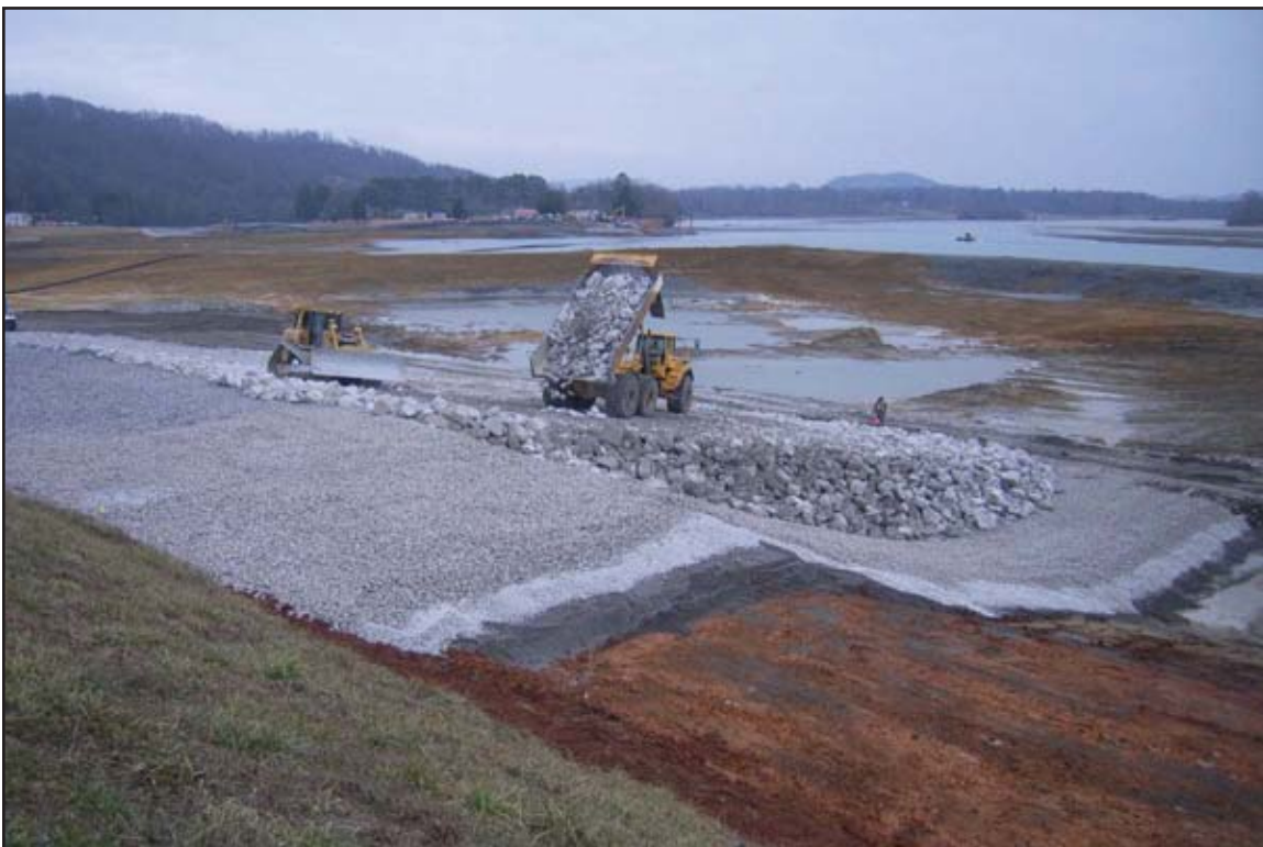
Progress of overall Dike C reinforcement work as viewed from top of Dike C. February 24, 2010.
