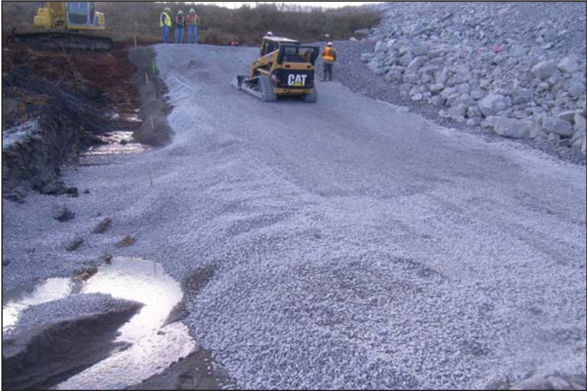
Placing layer of gravel on top of sand material in panel. December 27, 2009.
