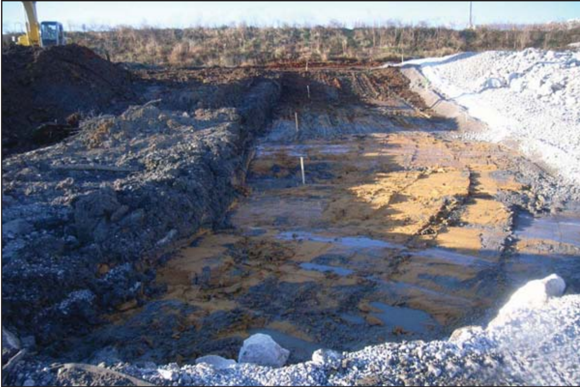
Excavating ash in “panels” from outboard slope of Dike C to expose dike material. June 5, 2010.
