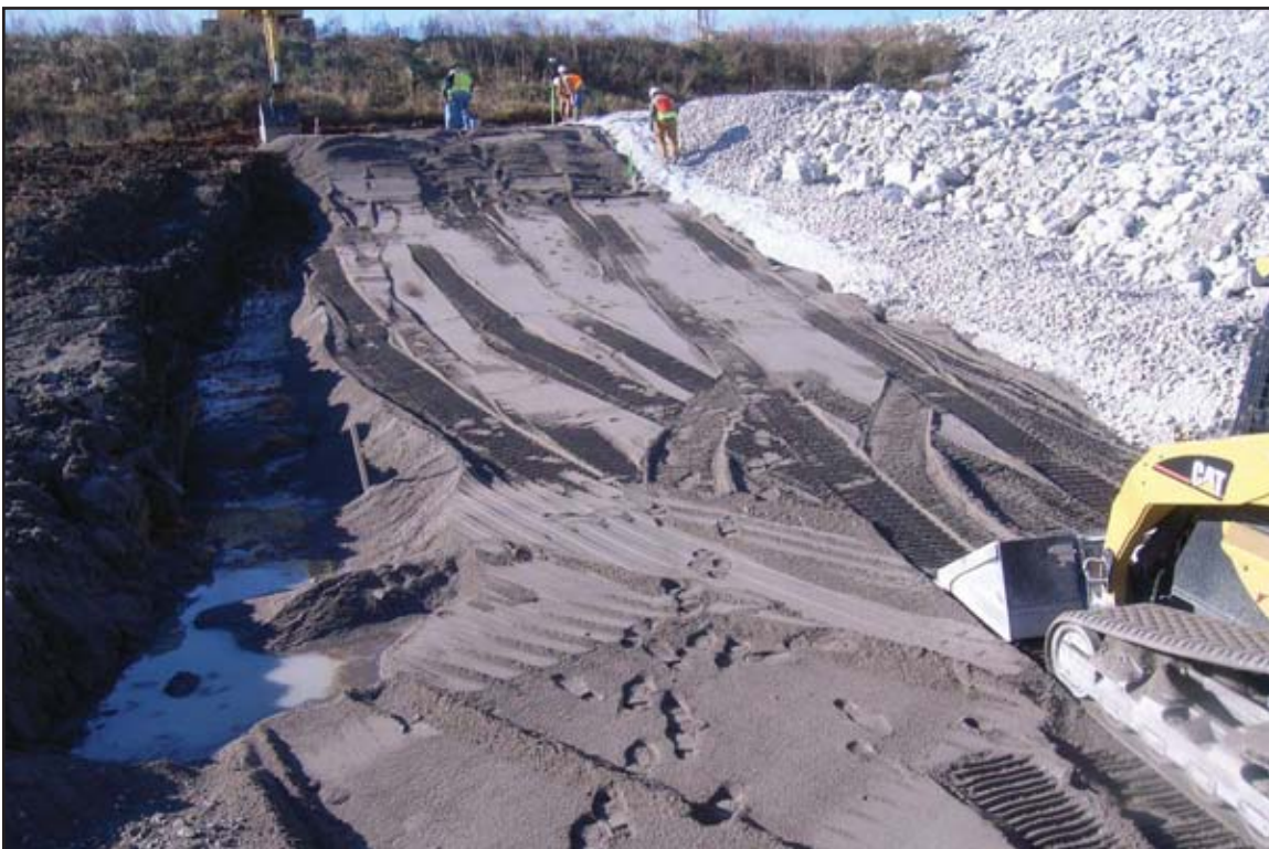
Placing layer of sand on top of dike material in panel. December 29, 2009.
