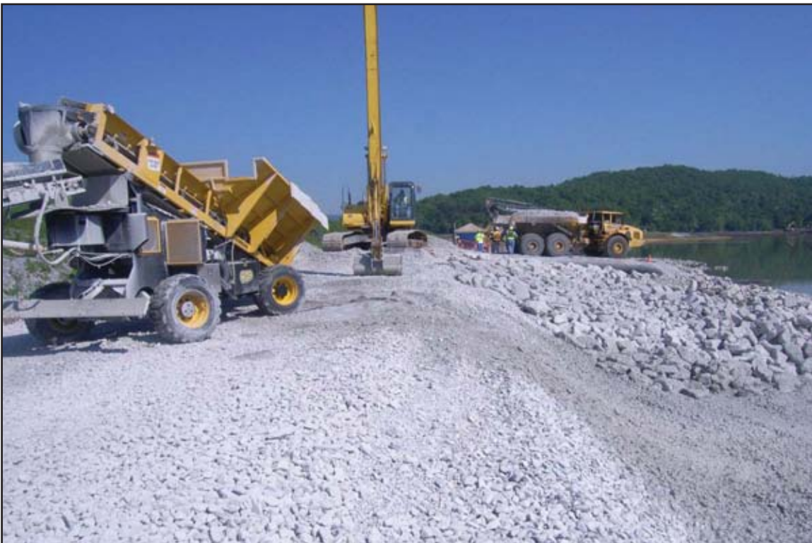
Equipment used in placing sand, gravel, and riprap during Dike C reinforcement. April 29, 2010.
