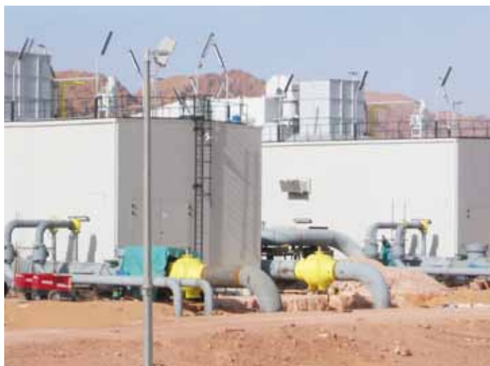
Hassi R'Mel Boosting Station, Algeria for Sonatrach
