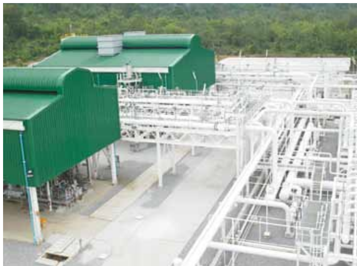
Saiyok Gas Compressor Station, Thailand for PTT
