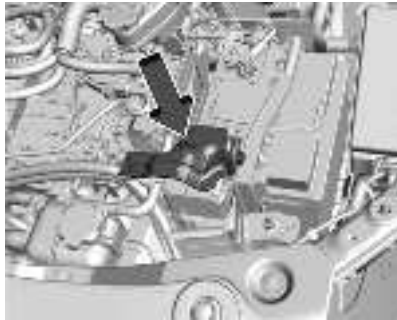
Discharged Battery Positive (+) Terminal
