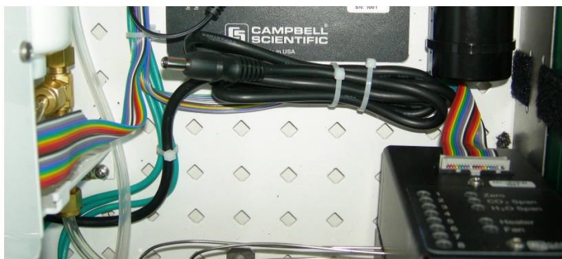
FIGURE G-2. Bundled cable of power adapter
