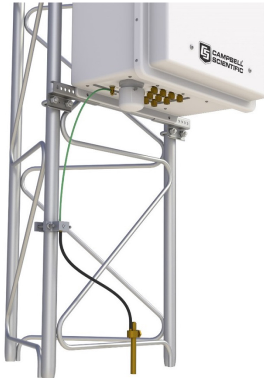
FIGURE 5-10. AP200 earth grounded on a UT30 tower
