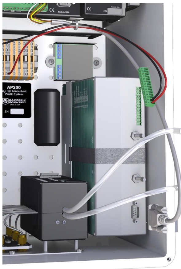
FIGURE 7-5. Components and fittings of IRGA installation
