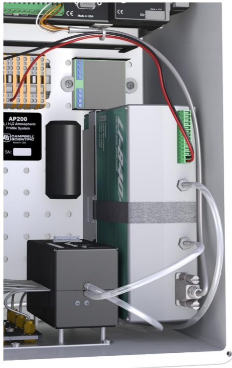
FIGURE 7-4. Installed IRGA in system enclosure
