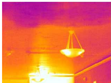
Leak in ceiling is nearly dry
