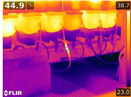
Failing electrical connector on a motor
