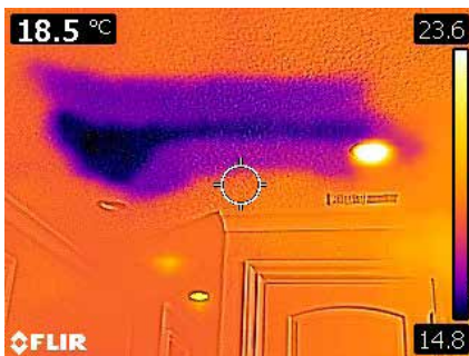
HVAC condensate overflow soaks a ceiling
