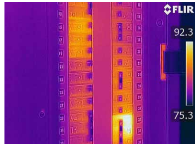
Overheating fuse in electrical panel
