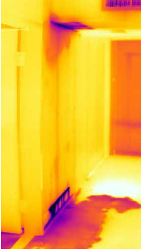
Water leak evident in a hallway
