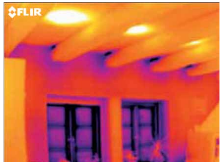
The thermal image shows thermal bridges between the roof beams and adjacent walls
