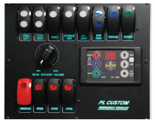
Conventional electrical and programmable thermostat in Life Support system
