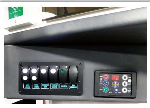
Auxiliary switch panel and thermostat curb side
