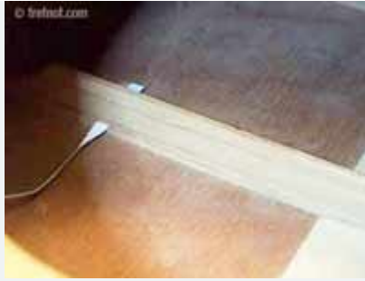
Paper strip shows location of a hidden crack
