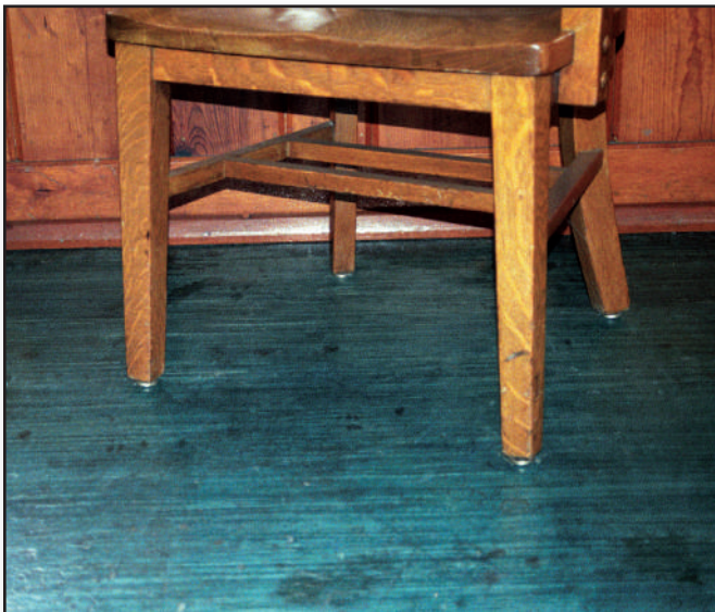
Figure 1—This jaspé pattern flooring has many dents and stains from years of use in the cookhouse at the Fenn Ranger Station (Nez Perce National Forest, Northern Region), but it is still serviceable.
