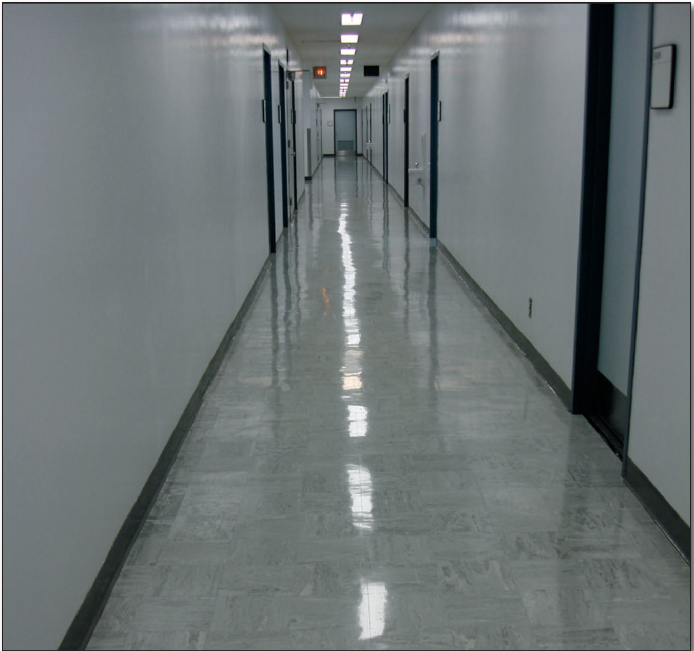
Figure 7—This vinyl flooring in the Intermountain Regional Office (Ogden, UT) has been freshly waxed and polished.
