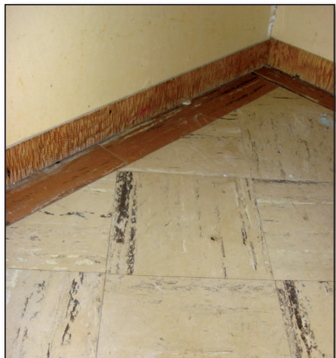
Figure 5—This asphalt tile flooring from 1951 has a darker band of tiles around the edge of the room for contrast and a plywood baseboard that was painted to look like the flooring.
