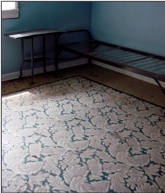
Figure 4—This intricately patterned, felt-base Congoleum “rug” protects the middle of the painted softwood floor of a bedroom at the Warm River Hatchery (Ashton-Island Park Ranger District, Caribou-Targhee National Forest, Intermountain Region). The Congoleum is in very good shape. The floor is spotted with flies that accumulated over the winter and have not yet been swept from the seasonal-use building.
