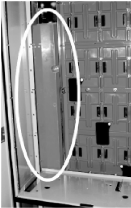
Bus Splice Access Cover In Place
