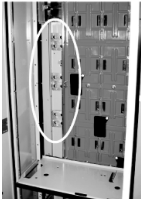
Bus Splice Access Cover Removed
