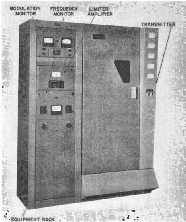
Fig. 8-3. A transmitter and associated equipment rack.
