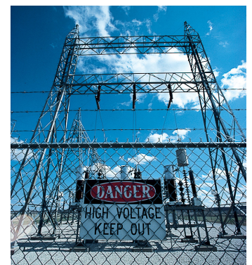
Utilities are increasing available fault current through installing lower impedance and larger kVA transformers.
