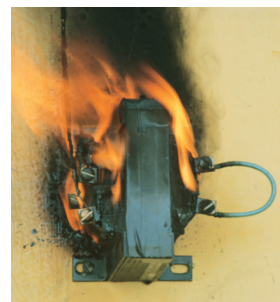
Figure 18: Fires can result if the correct OCPD amp rating is not applied.
