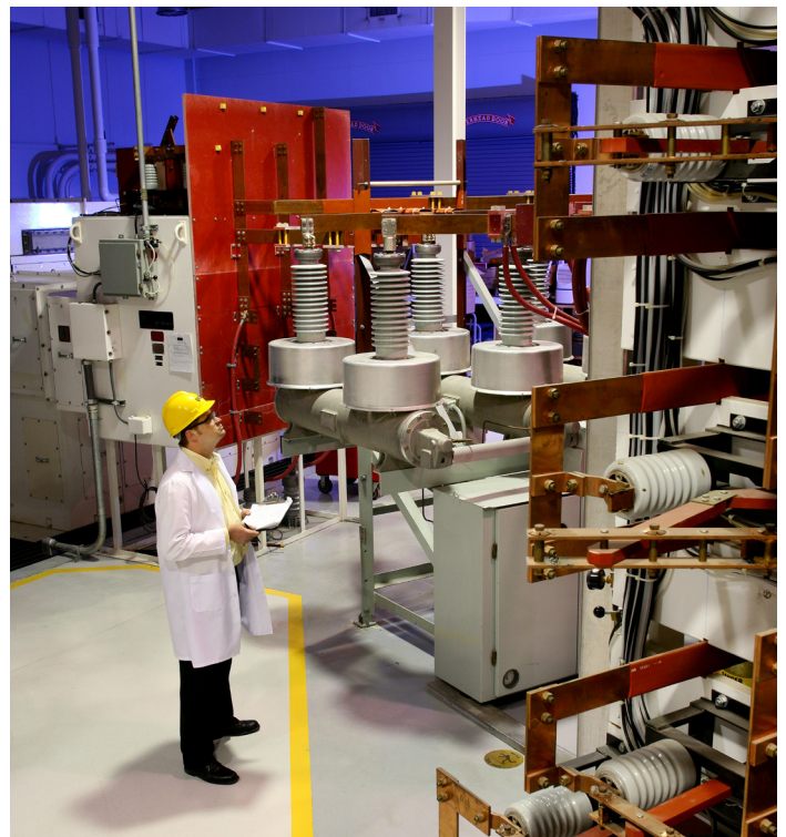
The Eaton Bussmann Division’s Paul P. Gubany Center for High Power Technology is the electrical industry’s most comprehensive facility for testing and certifying device and equipment SCCRs. Capable of performing electrical tests up to 600 V three-phase, 300 kA of short-circuit current for meeting ANCE, ANSI, CE, CSA, ETL, IEC and UL testing requirements.
