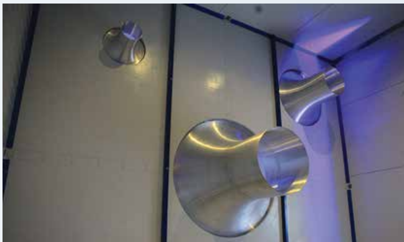
Air Flow Chamber, India.
