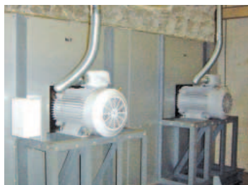
Air conditioning facilities at Kohda TEC
