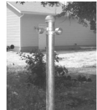
Proper installation of rail end cups and brace bands for a corner post. Notice one points up, the other down. This allows top rail to remain even at such a junction.
