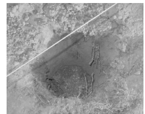
Fill post holes with concrete mix. Do not fill holes completely. This may cause posts to heave prematurely.
