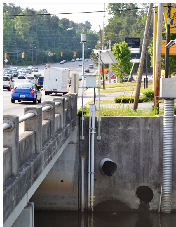
The GIL-B Monitoring Station
