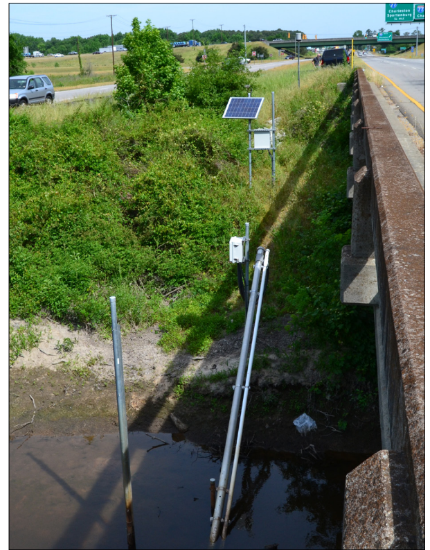
The GIL-C Monitoring Station
