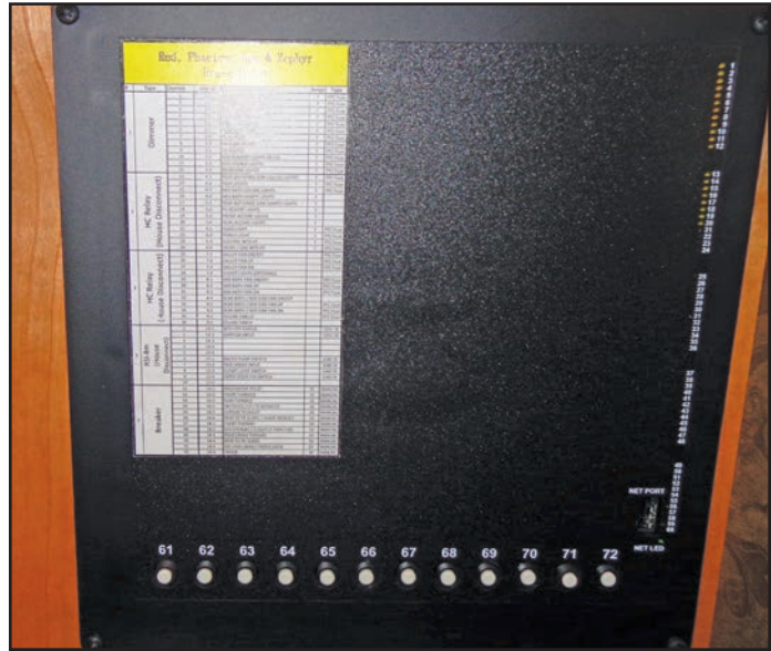
Figure 8-1: Circuit breaker box
