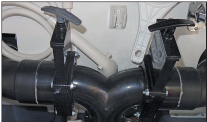
Figure 12-10: Sanitation coupling, valve and hose
