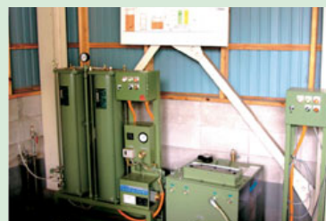
Cleaning liquid waste treatment facility
