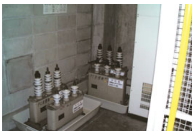
Storage of PCB waste
