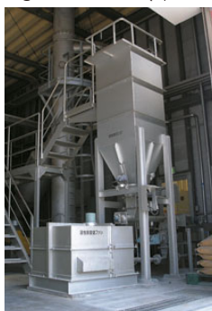
Activated carbon adsorption facility
