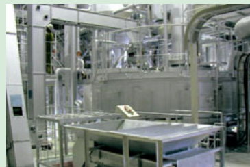
Green sheet waste recycling facility
