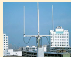
G3 base station
