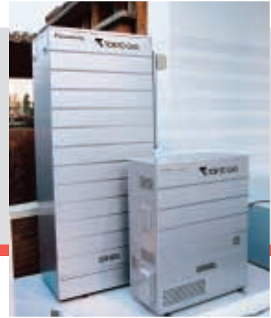
The world's first commercial household fuel cell cogeneration system was installed in the new official residence of the Japanese Prime Minister in April 2005.
