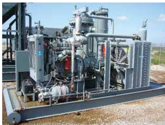
Figure 3.1 — A radiator cooling a G3304 NA Gas Compression Engine (at left). Note the second fan and cooler for the compressor gas near the rear of the package.
