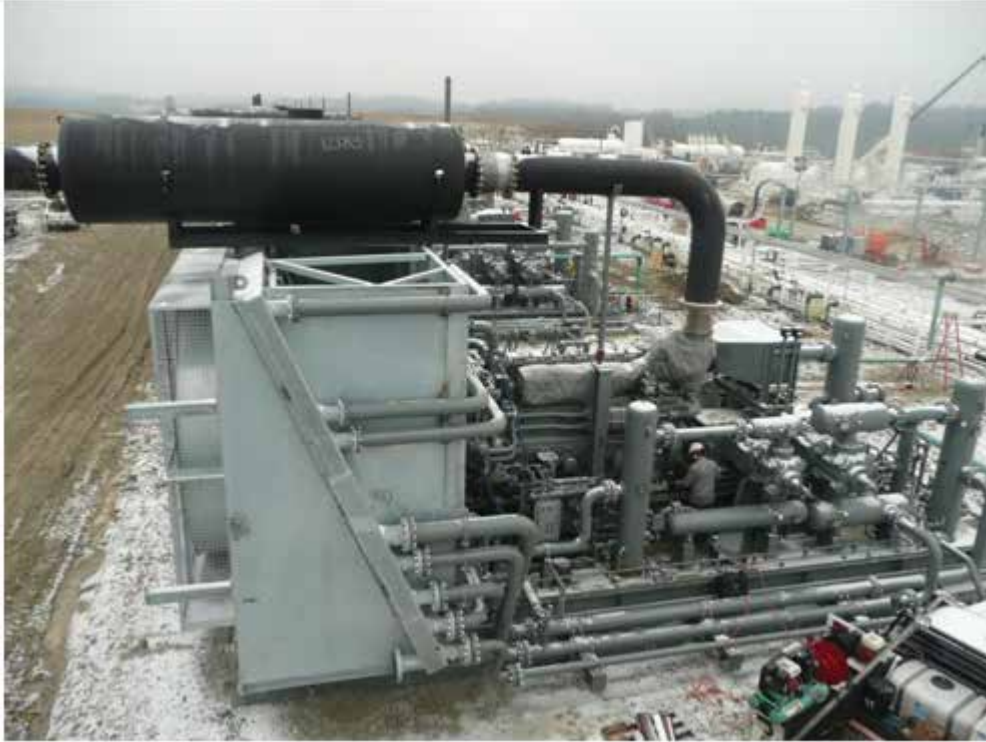
Figure 3.5 — Gas compressor package with vertical air cooler. For a size reference, note the service technician directly beneath the exhaust stack at engine rear.
