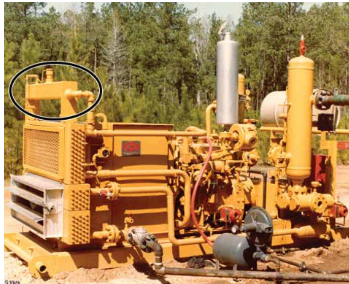
Figure 2.4 — An expansion tank on top of the cooler for a G3304 NA Gas Compressor Engine package. Only one tank is present because the engine is naturally aspirated, which means it will only have the jacket water circuit to cool. The other sections of the cooler are used by the compressor.
