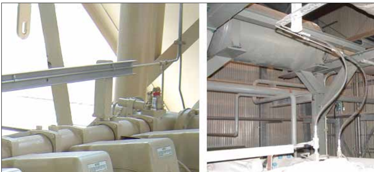
Figure 2.16 — Vent line installations showing both hard tubing and flexible hose in use.
