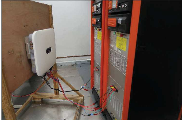
SURGE TEST (DC Main)
