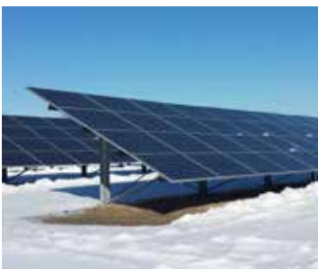
➤ Solar panels installed at Verizon facilities in Billerica, MA.
