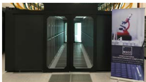
Singapore's National Supercomputing Centre
