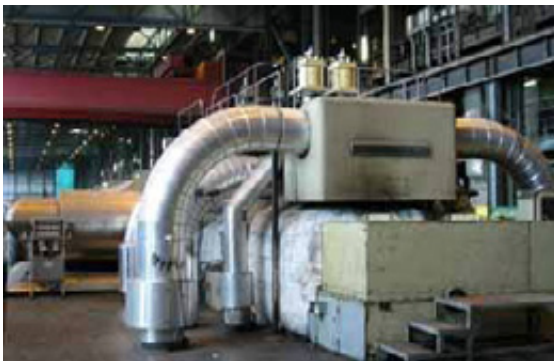
Figure 5.9 – CPT Blénod Power Plant Units 3 & 4, EDF, France
