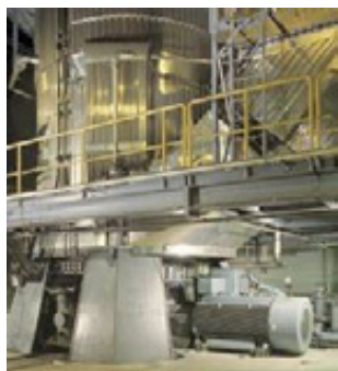
Figure 5.19 – Coal pulverizer with motor, (ABB Motors, 2006)
