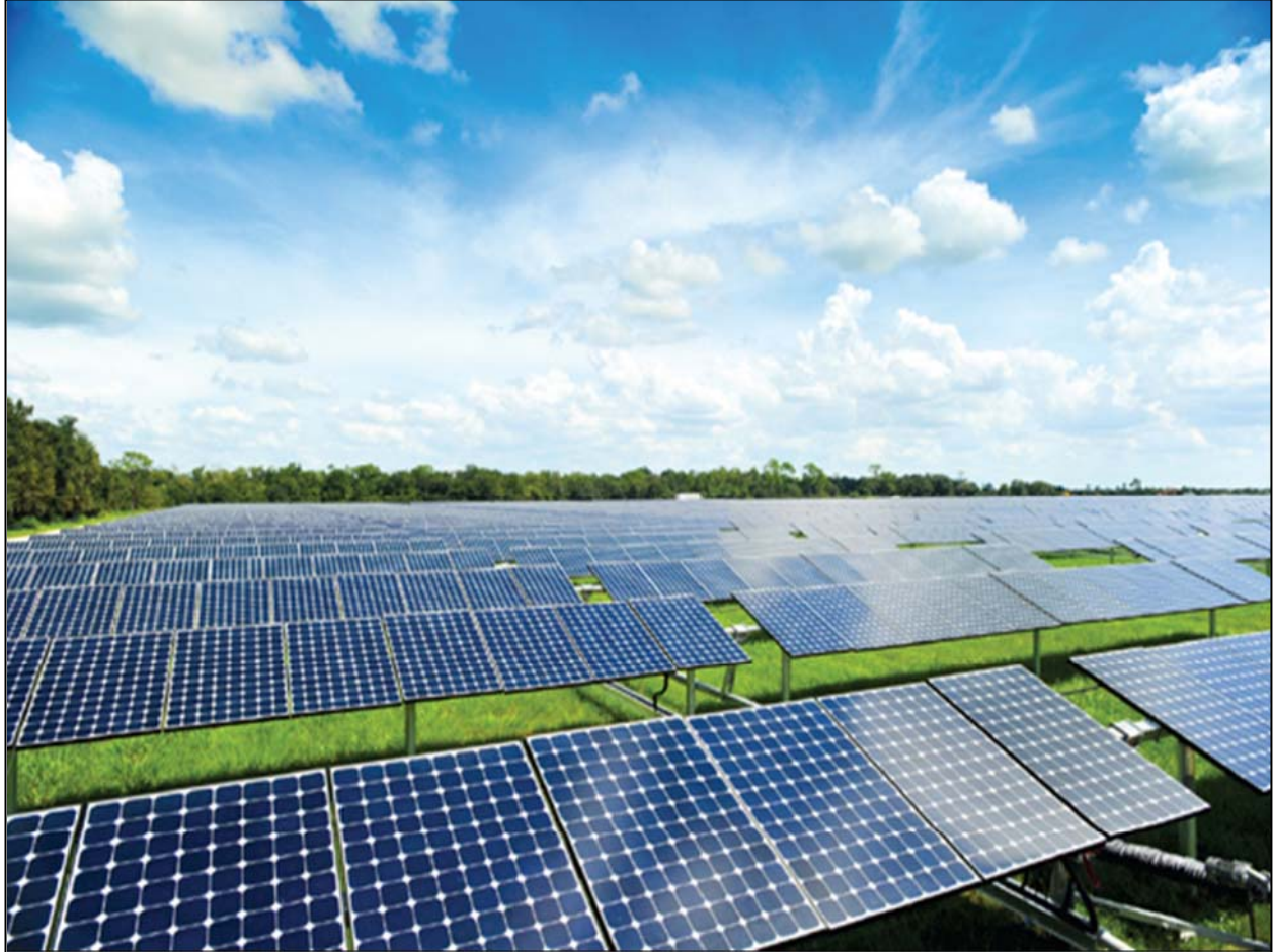
Photo 3.5-9. Single-axis, tracking photovoltaic system with panels close to maximum tilt.
