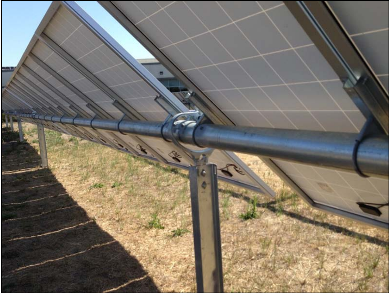
Photo 3.5-10. Typical view of the back of the solar panels.
