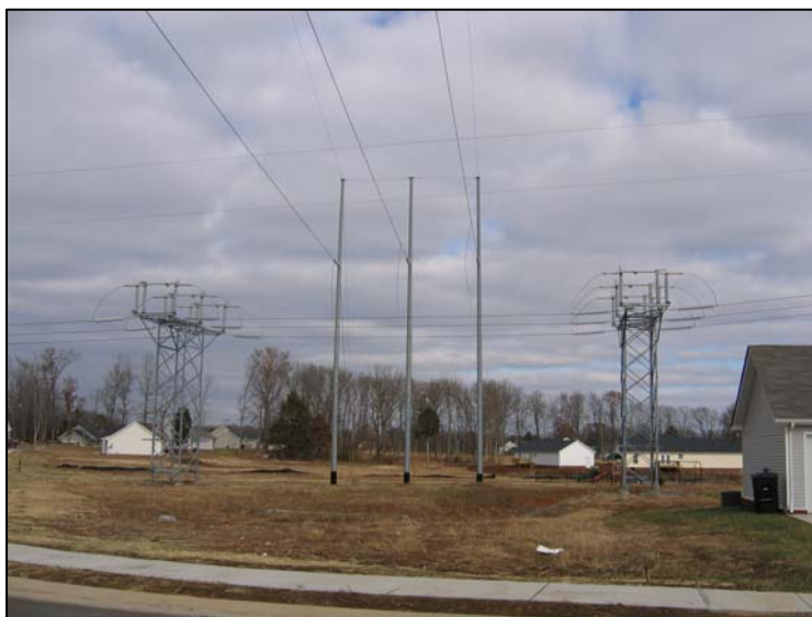
Photo 2.2-3. Example of switch structures and associated 3-pole transmission structure at a transmission line tap point
