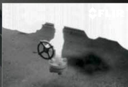
METHANE LEAK AT NATURAL GAS FACILITY SITE
