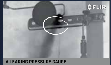
A LEAKING PRESSURE GAUGE
