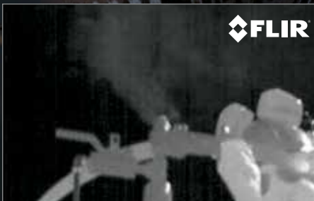
COMMON SF 6 PLUMBING LEAK
