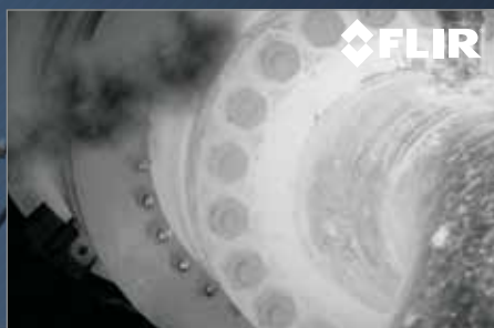
NATURAL GAS LEAK ON COMPRESSOR VALVE
