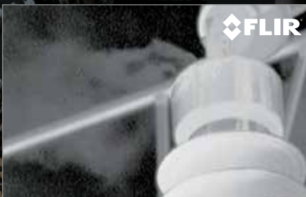
SF 6 LEAKING FROM CIRCUIT BREAKER
