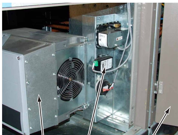
SUPPLY FAN VFD DUCT STATIC TRANSDUCER CONTROL COMPARTMENT
