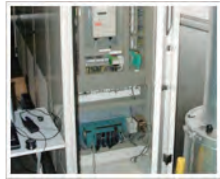
STARDOM controller installed in the site cabinet
