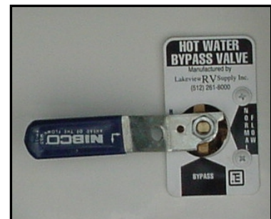
Figure 11-7. Water Heater Bypass Valve
