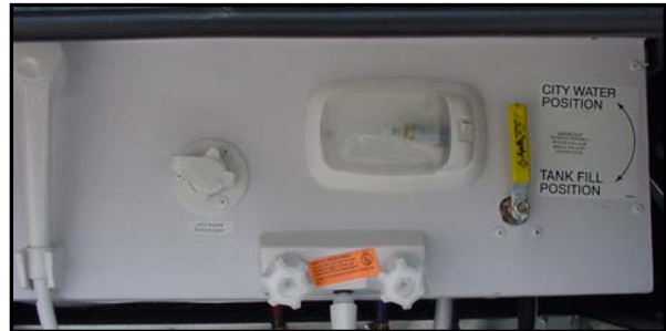
Figure 11-5. City Water Connection
