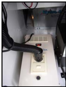
Figure 14-10. Vacuum Cleaner System
