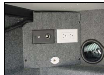
Figure 4-15. Cable & Telephone Jack
