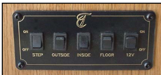
Figure 7-4. Battery Disconnect Panel
