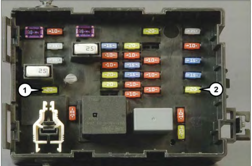
Power Outlet Fuses
