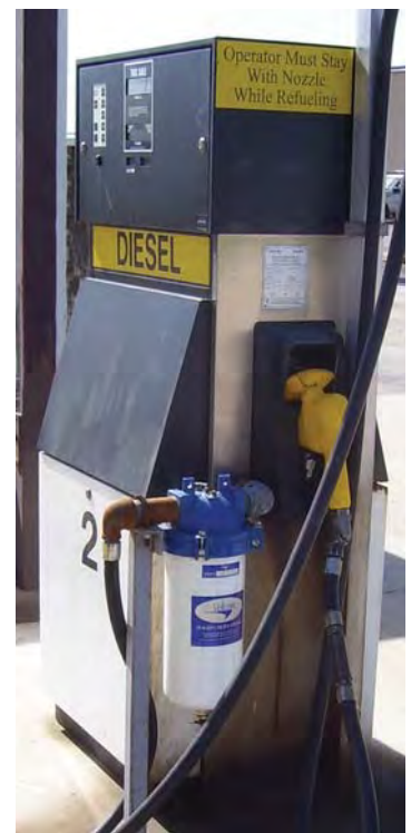
VF-61 connected to a diesel fuel dispenser
