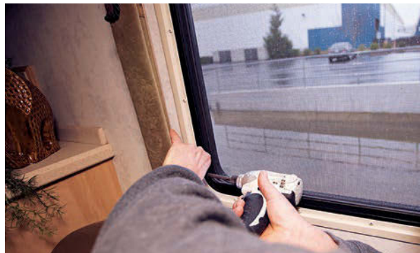
Strings that regulate the day/night shades were removed before the valances could be unscrewed from the walls. Measurements for the new shades were taken before the valances were removed.
