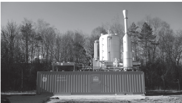
Figure 7 CHP in Augsburg.
