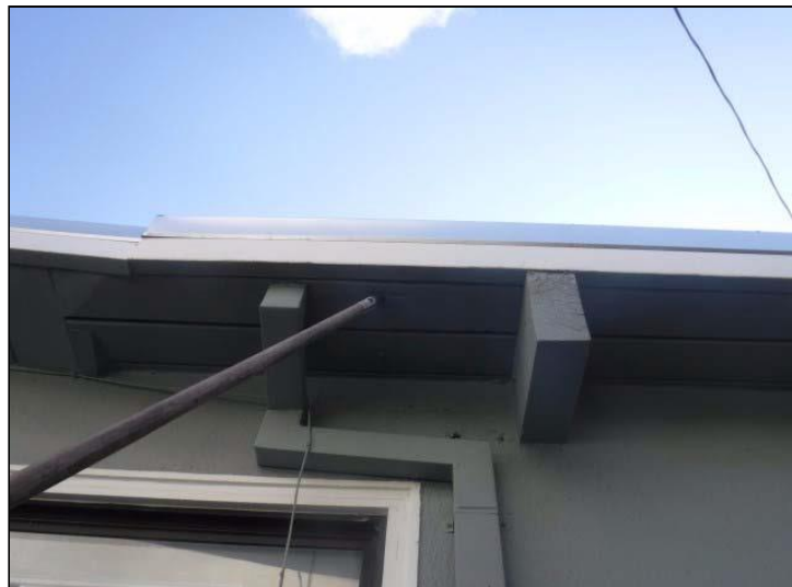
Location and Samples: Fungus Damage
