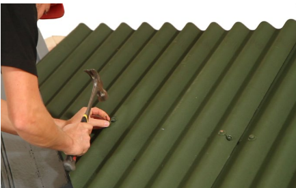
Fixing sheet to valley The fixings to the roof sheets can then be applied.
