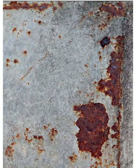
2 Steel structures are prone to deterioration in many environments.
