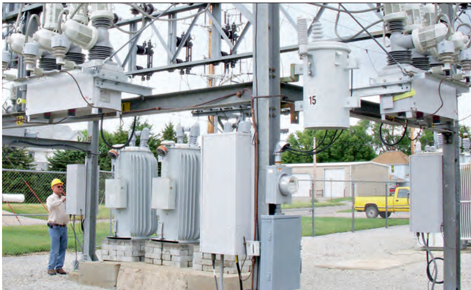
1 An ABB GridShield® recloser with RER620 in a substation
