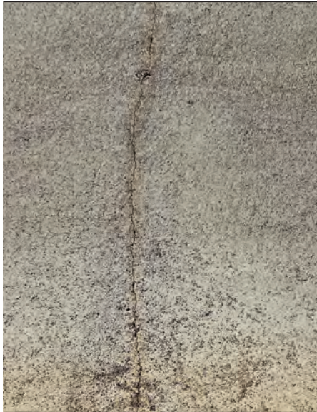
1 Concrete structures are susceptible to damage during transport or from manhandling.
