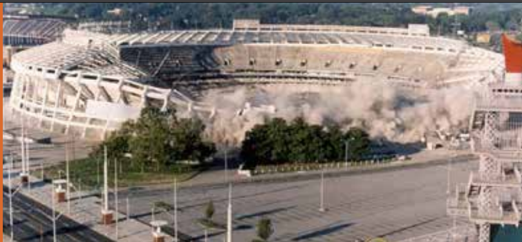
The Fulton County Stadium in Atlanta, Georgia, was imploded in 1997 – just 32 years after it was built and shortly after it had been refurbished to host the baseball events for the 1996 Olympics. It is a clear example of premature demolition because the building could not meet changing needs.
