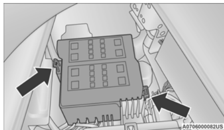
Rear Cargo Fuse Panel Cover
