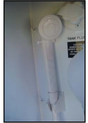
Figure 11-12. Exterior Shower and Exterior Light
