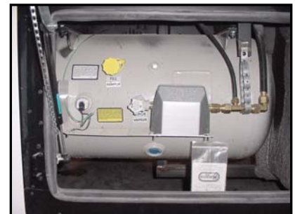
Figure 3-4. Liquid Propane Tank
