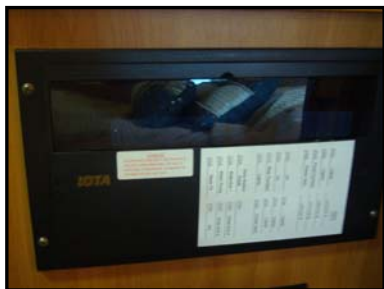
Figure 7-1. Circuit Breaker Box
