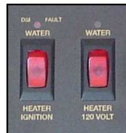
Figure 4-16. Water Heater Switches
