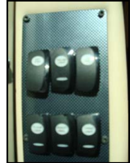
Figure 9-7. Entrance Step Switch (right middle)
