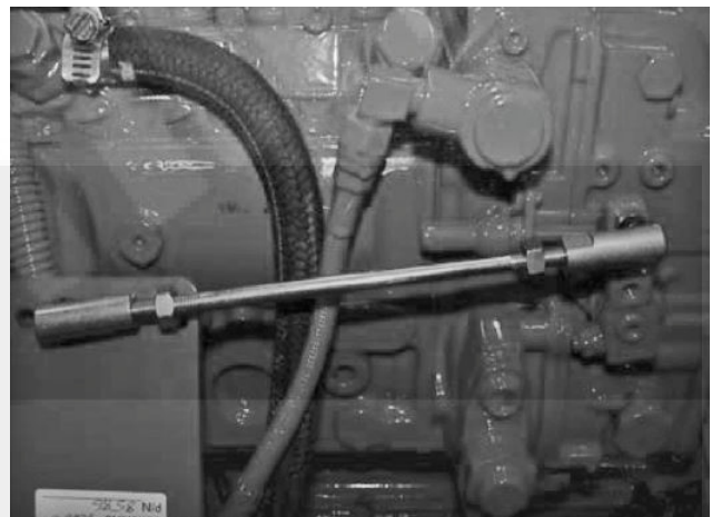
Figure 5-3 Fire pump drive engine linkage rod
