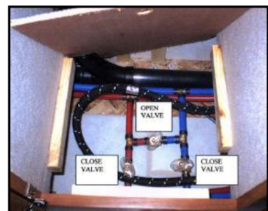
Figure 11-7. Water Heater Bypass System
