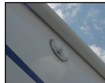
Figure 9-3. Security Light on Exterior
