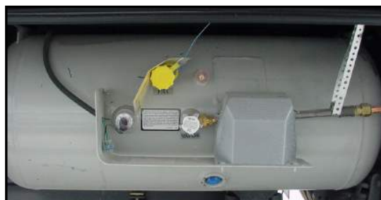
Figure 2-2. Liquid Propane Tank
