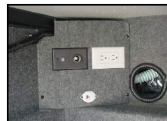
Figure 4-14. Cable & Telephone Jack
